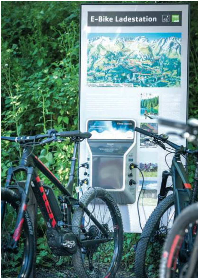
Encouraging e-MTB tourism requires installing charging station along popular routes. (Photo: Gaudenz Danuser)
